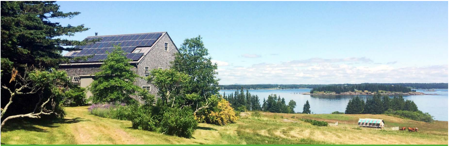
A rooftop array perched on a coastal hill on the island of Vinalhaven in Maine. Photo credit William Byers.
