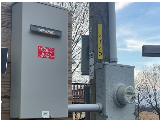
This automatic transfer switch acts as a safety gate—ensuring generator power never feeds back onto utility lines and keeps crews protected while they work.
